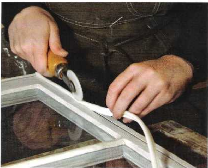
Figure 4. The author prepares a sash to receive weather stripping by routing a 3mm groove into the mating surfaces of the sashes (top). After the sash is fully primed, horizontal surfaces — such as the meeting rail shown above — are fitted with silicone bead. On the exterior of each sash, vertical surfaces are fitted with brush-type weather seals, which seal tightly to the stops but don't interfere with opening and closing.
