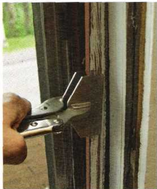
Figure 1. A set of wide-mouth Vise-Grips helps extract parting bead without undue damage.
