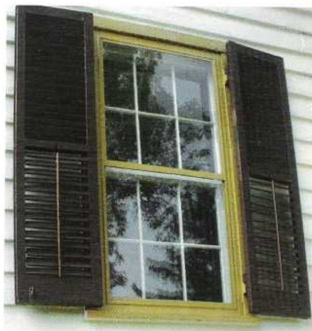
Figure 6. A restored double-hung's authentic divided lights and period glass are visible even behind a storm window. With occasional maintenance, this unit should serve faithfully for another century.
