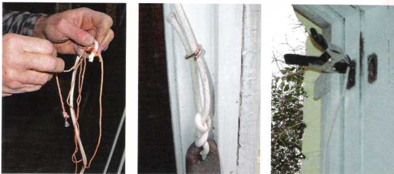
Figure 5. A weighted string helps the author fish new sash cord over the pulley and down to the bottom of the weight box (left). He secures the cord to the sash weight with two half-hitches, then captures the excess cord with a hog ring to prevent it from ever getting snagged in the cavity (center). To allow plenty of slack for attaching cord to sash, he pulls the weight to the top of the cavity and clamps the cord (right).
