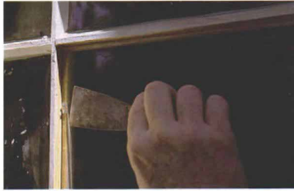
Glazing points are pushed in with a putty knife. With the glass set in the frame, glazing points are inserted to keep the pane in place. Tiny vertical tabs on the points let you use a putty knife to push the points into the wood.
