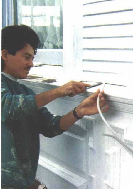
Filling wide cracks. Backer rod is a compressible foam rope that can be squeezed into a crack too wide to caulk. Once in place, the remainder of the crack is filled with caulk.
