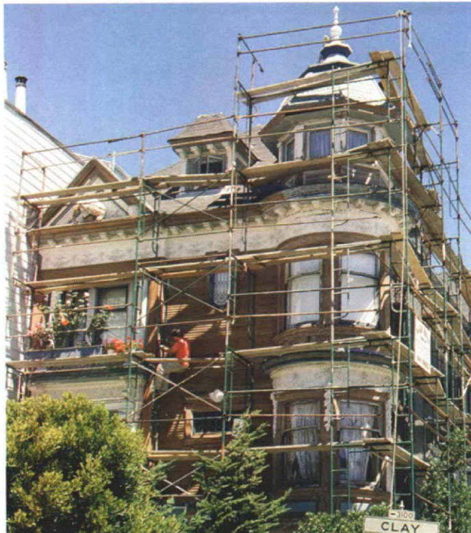
Almost a century old, this Queen Anne Victorian house is decorated with redwood trim and plaster garlands. A job of this scope begins with a thorough cleaning done from a scaffold that allows access to every exposed portion of the building.
