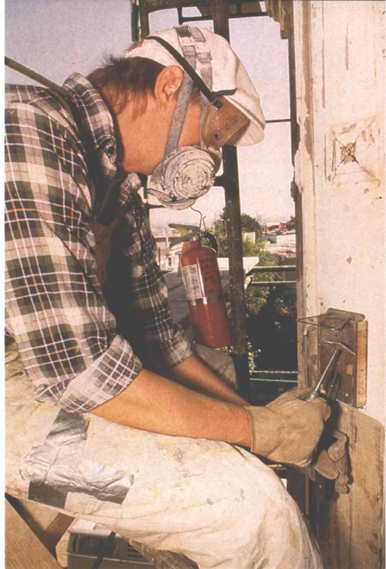
A heat plate is an electric paint remover that softens paint without an open flame. This method avoids the hazards of burning paint scrapings falling around the base of the building.
