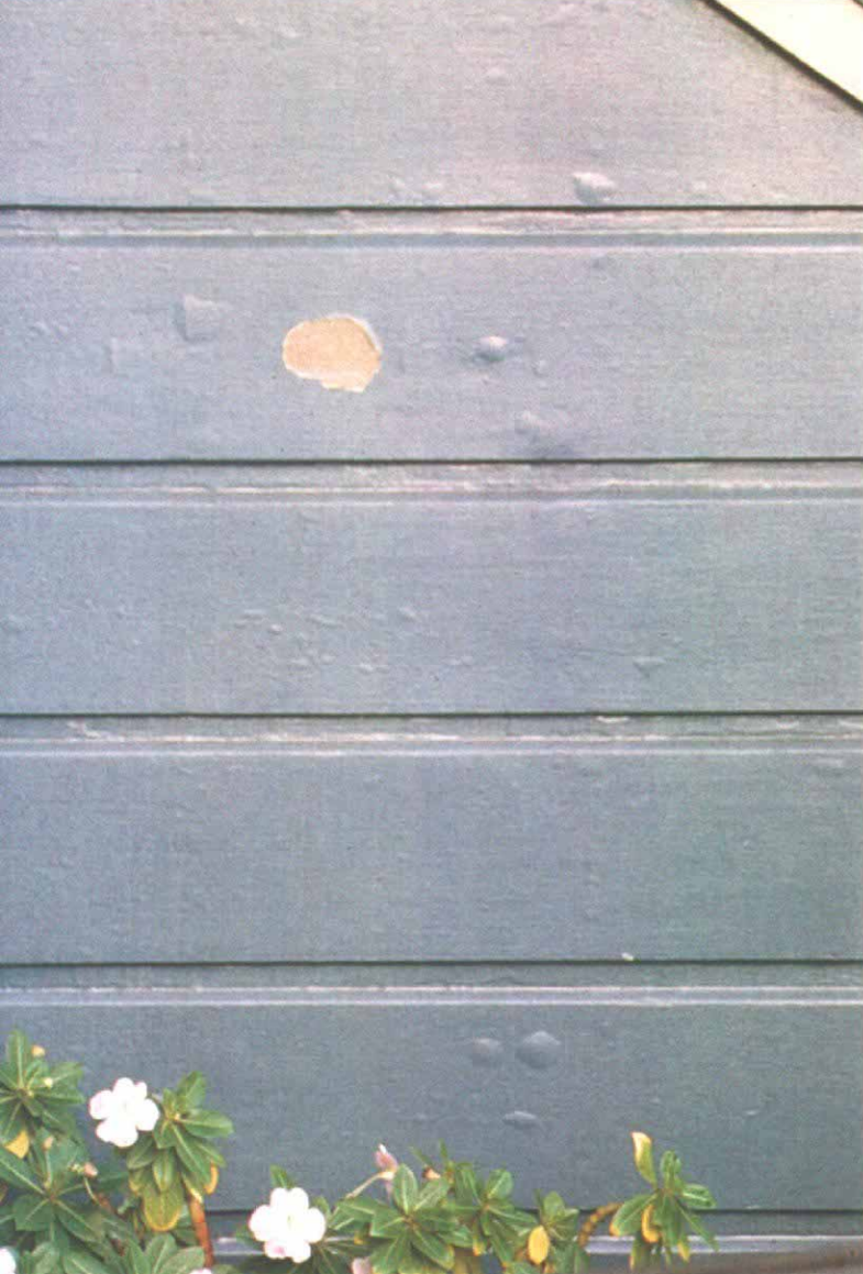
Failure. Once paint has started to blister, you can be sure that the bond between the first layer of paint or primer and the wood has failed. When this happens, it's best to take the surface back to bare wood.
