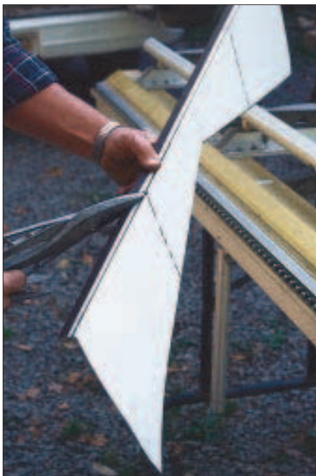
Figure 5. The author cuts pie-shaped pieces in the folded hem so that the counterflashing can be bent around the chimney corner.
