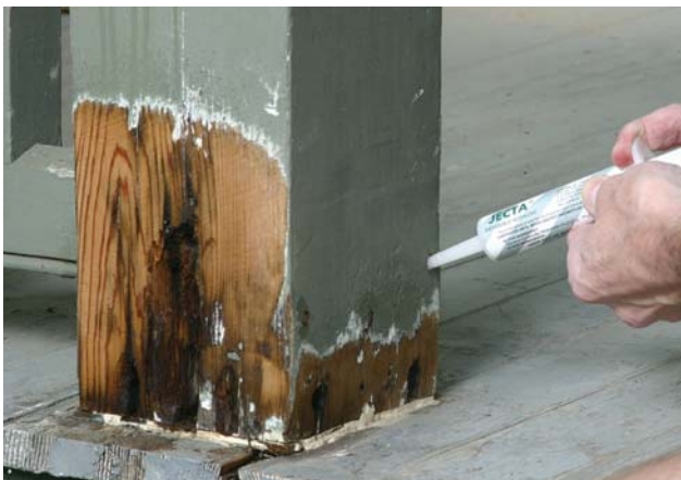
Figure 1. A painter's 5-in-1 is the perfect tool to carve into rot-damaged wood and excavate the black, punky detritus (top). After the worst of the damage has been removed, a solution of powdered borate and water is sprayed on the affected surfaces to kill the rot organism (center). To quickly attack deeply buried rot, a borate gel is injected into a few small holes that have been drilled into the center of the wood (above).
